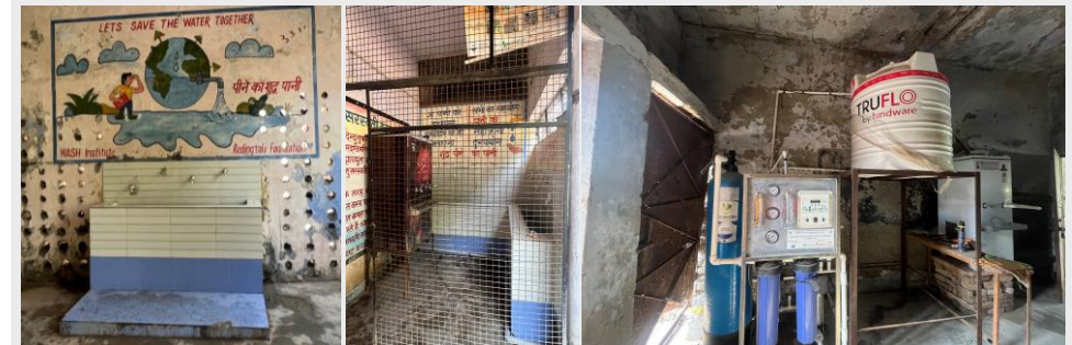
Height appropriate drinking water stations with water cooler and filtration system
