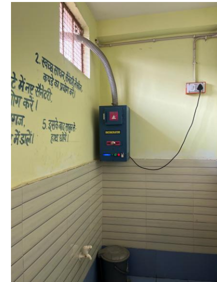
Incinerator in the changing room at Government School, Chhainsa
