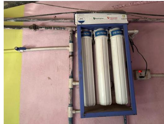
Water Filtration system at Khaskhamar High Madrasah, Uluberia
