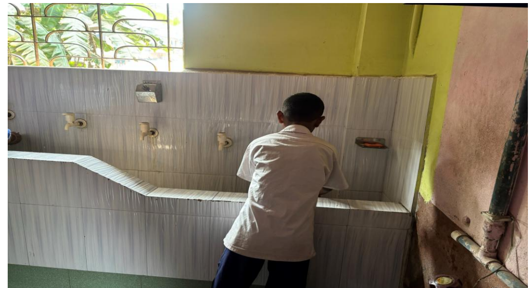
Height appropriate handwashing station at the school
