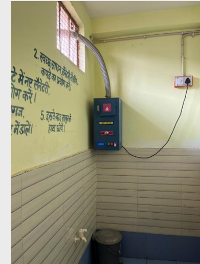
Changing room for girls with incinerator
