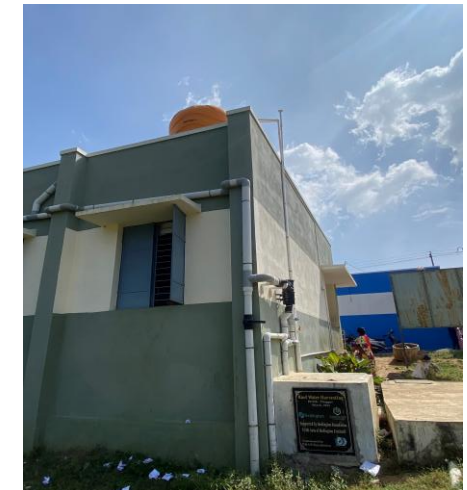
Rain Water Harvesting installed in schools
