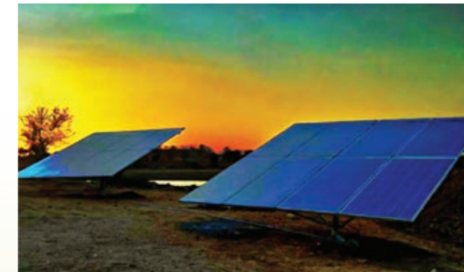
Solar Panels installed for a small business in UP.
